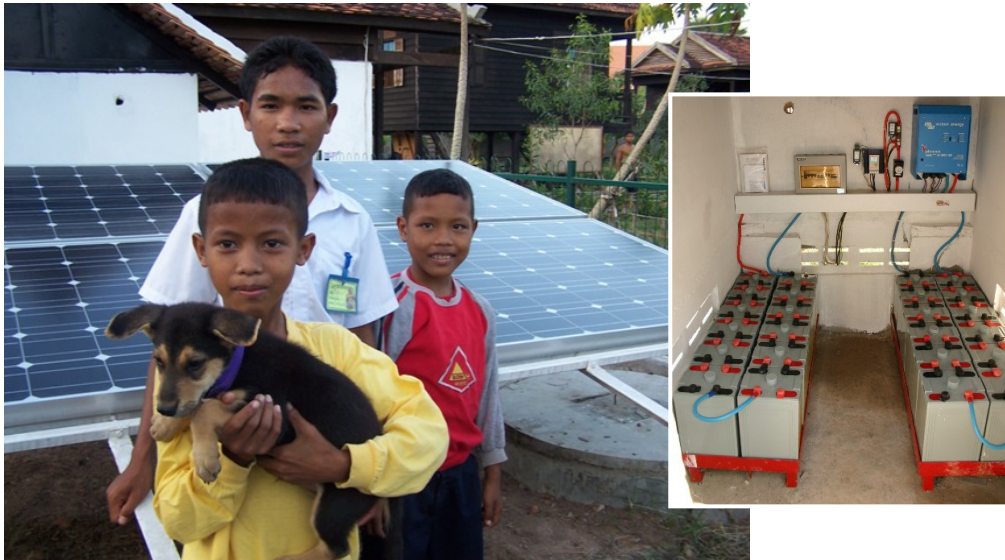
▲ Solar power system at Cambodian orphanage. About 70 children have enough power for lighting. Also a television and a computer is connected to the system. Inset: The inner part of the technical area provides space for batteries, a controller and inverter.
